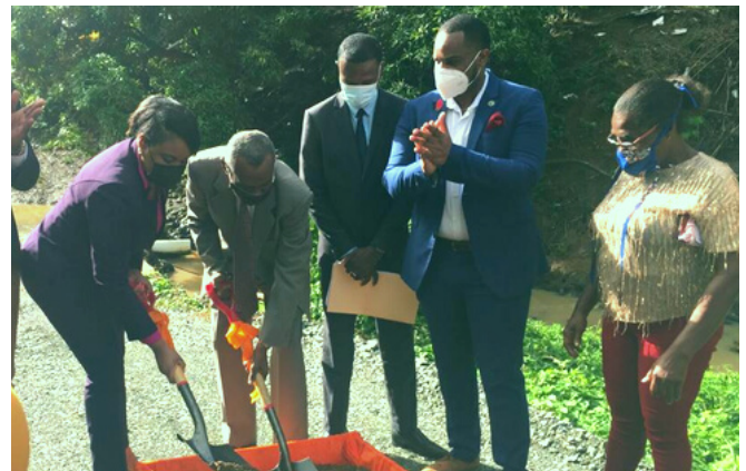
Minister Shamfa Cudjoe and Chairman Anthony Campbell turn the sod for the Grandy Gully Bridge. Looking on are CEO Elroy Julien, Mr. Kwesi Des Vignes and residents.
